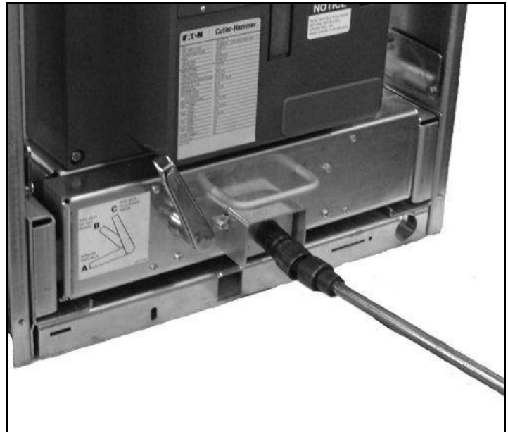
Figure 4-17 Levering Circuit Breaker
