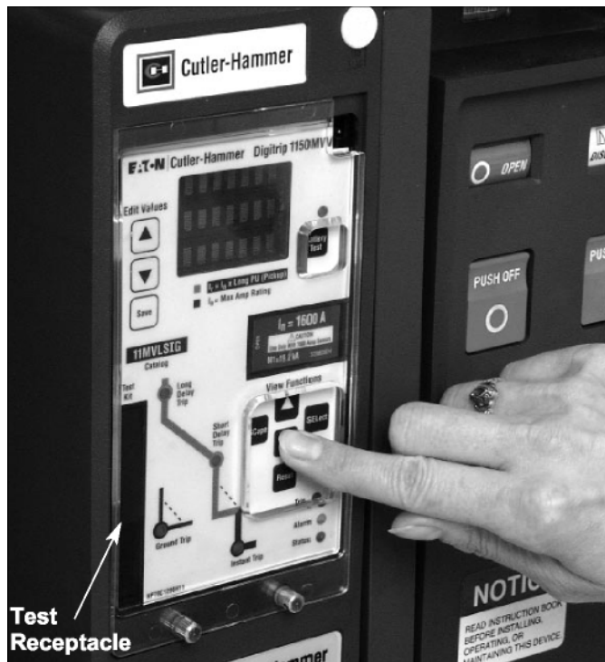
Figure 5-19 Digitrip RMS 1150 Vi Programmable Trip Unit Installed in T-VAC Circuit Breaker
