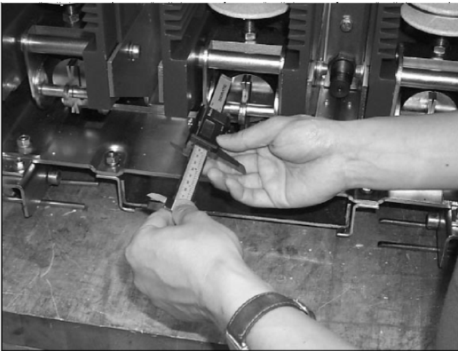
Figure 6-5 Contact Wipe Measurement Being Taken on Middle Pole of Closed 40kA Breaker
