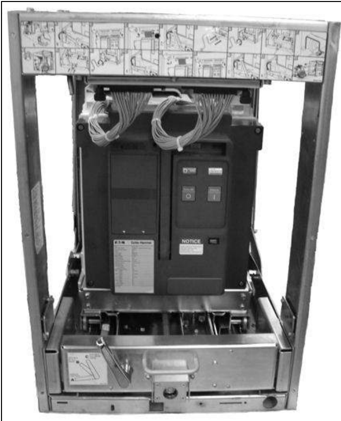
Figure 4-19 Circuit Breaker Shown in CONNECT Position with Secondary Connections Made
