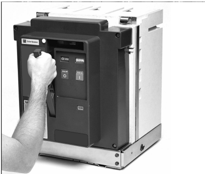
Figure 5-6 Breaker Closing Springs Being Manually Charged
